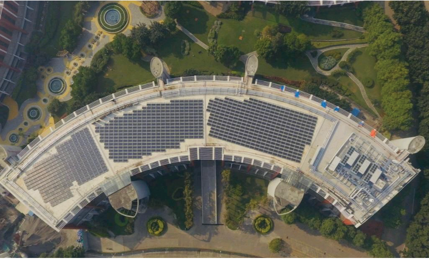
Solar Power Plant (rooftop and ground-mounted systems)
