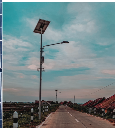
Solar Street Lights
